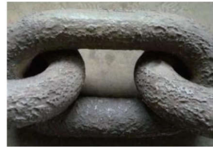
腐蚀状态分析 Corrosion analysis
