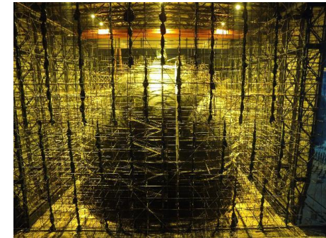
Insulation under shelter 风雨棚内绝缘
