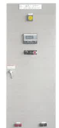
[ Self Standing Control Panel ]
